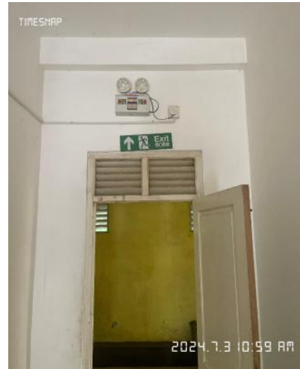
34. Emergency Lights at dormitory.JPG
