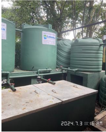
29.Waste water treatment plant.JPG
