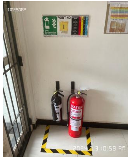
32.Fire Extinguishers at dormitory.JPG
