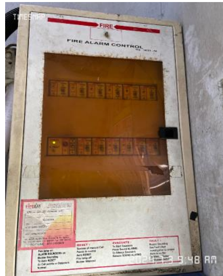
12.Fire panel board.JPG
